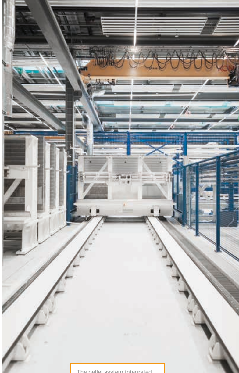
The pallet system integrated by the Starrag Group includes a total of 16 pallets measuring 2,000 mm x 4,000 mm.
