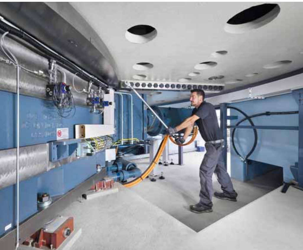
Easy access: The basement across two stories enables easy and ergonomic work on all machine assemblies and supply units.
