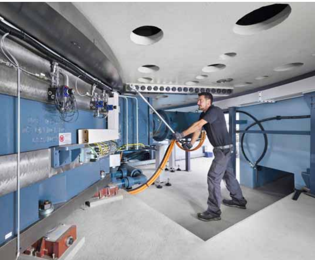
Easy access: The basement across two stories enables easy and ergonomic work on all machine assemblies and supply units.
