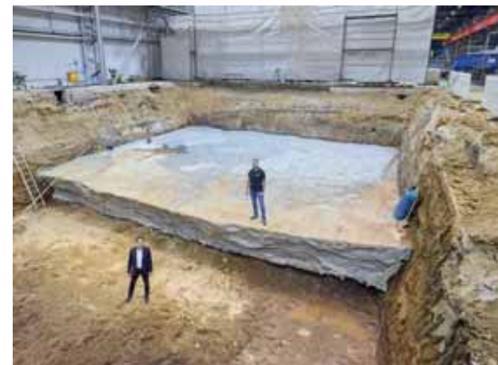
Preparations are underway for a foundation to accommodate a new Droop+Rein FOGS HD large-scale machining centre, which will be built in autumn.
