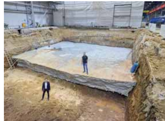
Preparations are underway for a foundation to accommodate a new Droop+Rein FOGS HD large-scale machining center, which will be built in autumn.
